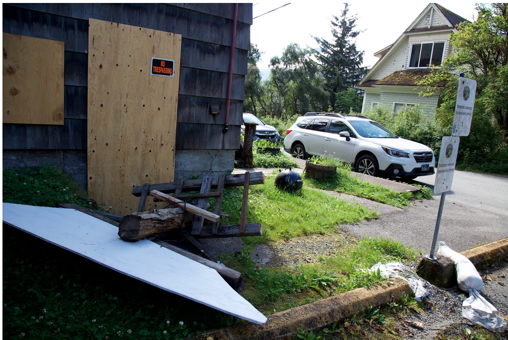
Boarded-up homes on Telephone Hill on Tuesday, Aug. 25, 2026. (Mark Sabbatini / Juneau Independent)
